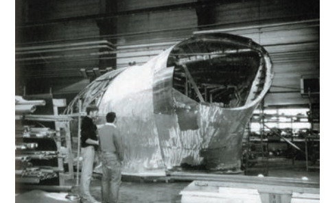
Design and construction of a form for the Restaurant Le Georges, Centre Georges Pompidou, Paris, by Jakob+MacFarlane sarl d'architecture (Schmal, 2001, 132-135)
