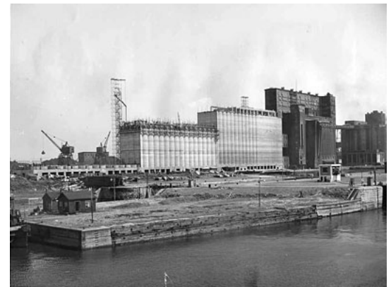
Fig. 8: Construction photo of the 'B-1 Annex' by C.D Howe. Source and date unknown.
