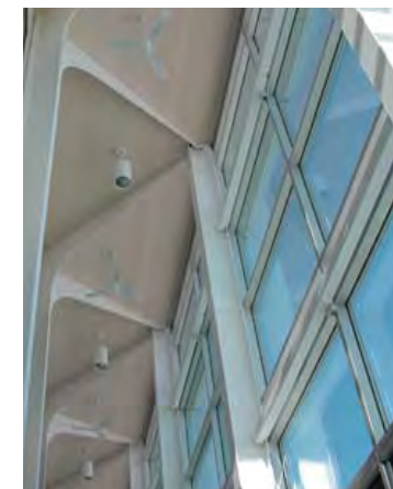
St. John Ambulance's Provincial Headquarters in Edmonton, Alberta was awarded a LEED™ Silver rating. The height of the east facing atrium/lobby was supported by an architecturally exposed structural steel system that used unique Y shaped columns, comprised of plate members, to support and provide character for the three storey energy efficient Vision Wall system.
