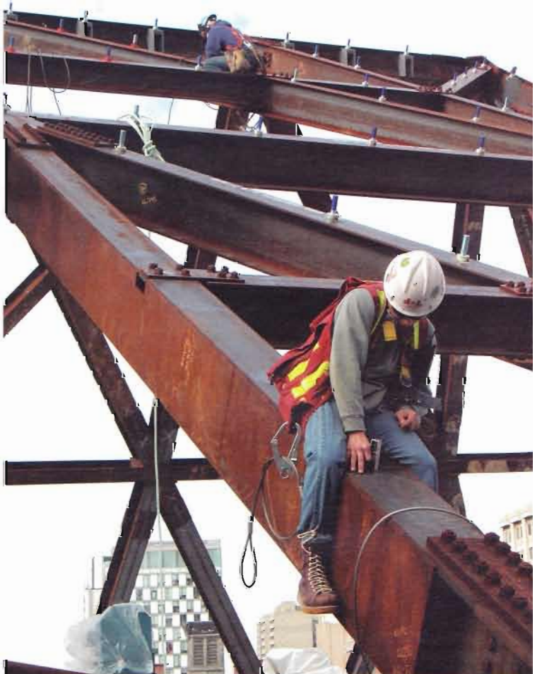
TOP A VIEW FROM INSIDE THE NEST OF CRYSTAL'S. RIGHT WORKERS INSTALLING SOME OF THE 10,000 CONNECTORS USED FOR THE EVENTUAL CLADDING SYSTEM.
