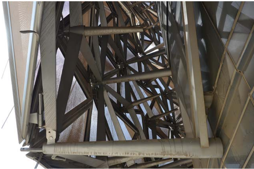
Figure 11: A view up through the double façade during construction. The transparency of the PTFE panels can be seen.
