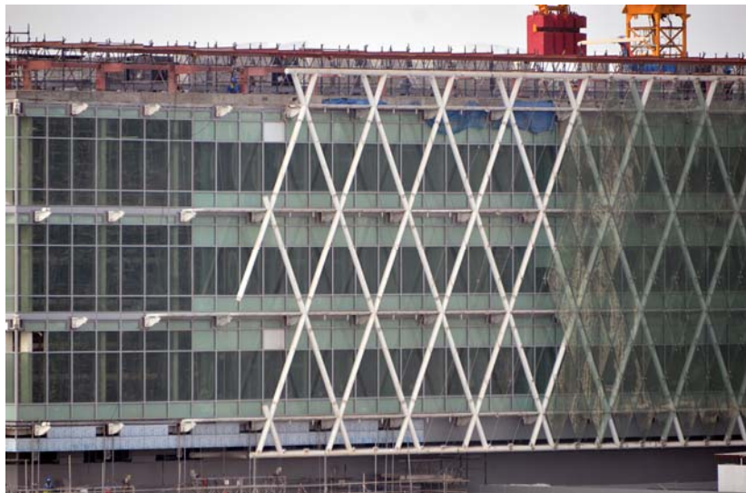
Figure 14: The installation of the layers of the double façade. The interior layer is a fairly standard sealed rectilinear curtain wall system. The tubular steel diagrid that supports the exterior layer of glazing is supported by arms that are connected back to the building structure. Grated walkways span between the arms to provide access to the cavity for cleaning and flow through ventilation to support the stack effect. The exterior diamond shaped glazing layer is connected to a cable system that is used to further subdivide the larger structural diamonds.
