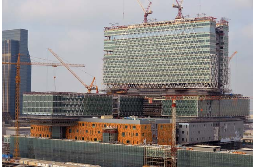
Figure 13: The Cleveland Clinic under construction in 2012. A hollow structural steel diagrid is used to support the exterior layer of the modified buffer system. The steel diagrid system was prefabricated in uniform modules allowing for a fairly rapid site assembly to take place.
