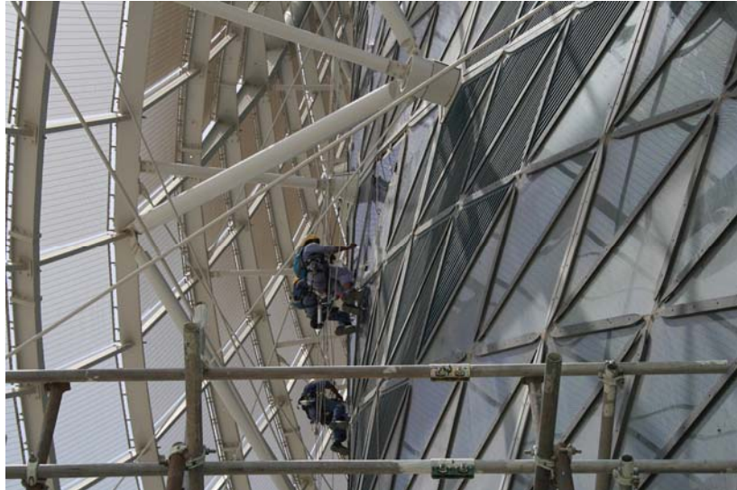
Figure 16: Abseilers clean between the curtain wall and metal "splash" (credit Jeff Schofield, ADNEC) and maintain the exterior of the double façade skin.
