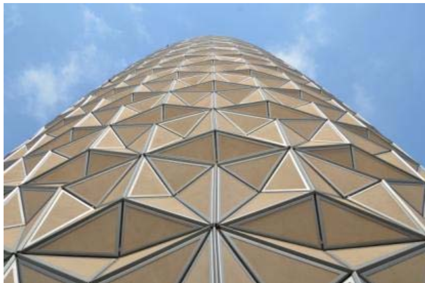
Figure 12: When the mashrabiya is in its fully closed position, the majority of the harsh desert sunlight is prevented from striking the glazed façade thereby reducing the cooling load on the building. Although the mashrabiya may appear very solid in this view, it is created from a PTFE screen material to allow some light to the interior.
