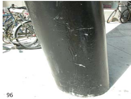
96 This thick intumescent coating is constantly being repaired due to its high traffic location as well as repeated incidences of graffiti removal. The colour matching on some of the supports is more difficult to achieve.
