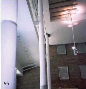
95 The colour and texture of intumescent coatings is not the same as normal paint so it is necessary to detail items like these columns to recognize that the finishes are not the same. Here a band of a different colour highlights the change.
