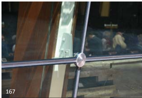
167 Although the interior of this lobby would give the appearance of being supported in heavy timber, here we can see that the framing is steel with wood cladding. This permits the connection of spider connectors to the steel structure hidden inside.
