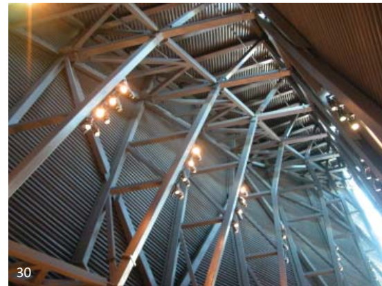
The Canadian War Museum in Ottawa uses AESS to create a highly articulated and rugged expression in the steel in Regeneration Hall. In this instance a combination of welded connections and exposed plate to plate moment connections at the connection points between square HSS sections is the feature of the appearance. Due to the irregularity of the structure, tight tolerances are required. The profiled decking is also left exposed to view.
