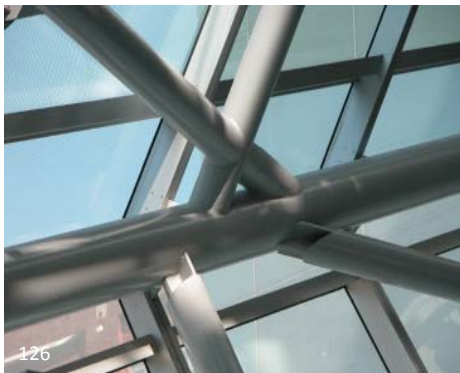
126 These tubular members were welded, using both tube to tube connections as well as X shaped plate fabrications to resolve the geometry of the transition.
