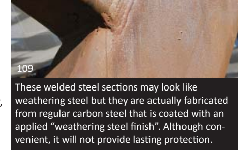
109 These welded steel sections may look like weathering steel but they are actually fabricated from regular carbon steel that is coated with an applied “weathering steel finish”. Although convenient, it will not provide lasting protection.
