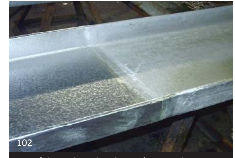
One of the technical realities of using galvanizing as a "finish" lies in the inconsistency of the product. The difference in this photo is due to finishing temperatures. If galvanizing is used as a final coating on an AESS project differentials in finish must be both understood and detailed into the project.
