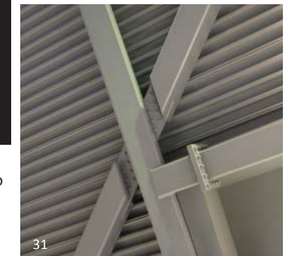
In the Canadian War Museum there are exposed welded and bolted connections. Square plates have been welded to the HSS members that provide surface for bolts on all sides of the connection to ensure a uniform appearance. Flat plates have been used for the lap type hinge connections on the diagonal members, creating a degree of uniformity within the scheme.
