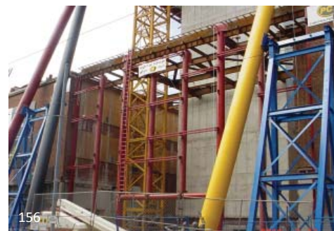
The blue frames are temporary supports that were constructed to shore up the sloped columns precisely, using padded support points as not to damage the intumescent coating that had been shop applied.
