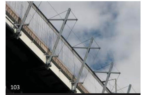
Galvanizing is a suitable finish for an exterior AESS structure that will be constantly subjected to weathering as in this expressive railing system.
