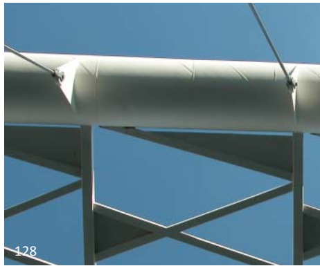
128 The large HSS members used on this bridge have helical welds. Although unusual in appearance, they were aesthetically worked into the design.
