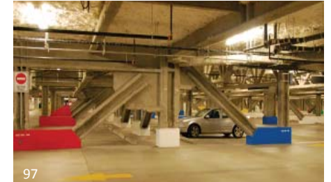
97 Cementitious finishes can be commonly found on exposed steel used in parking garages. While not falling in a regular AESS category, care has been taken here with the design of the support system in the garage.
