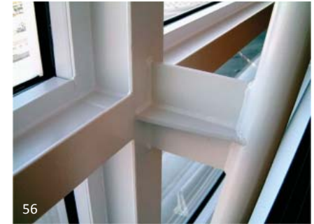
56 Fig. 2.4B Welds are plainly visible but of good, uniform quality so complementary to the structure.
