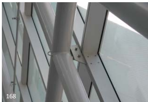
168 This tubular steel framing system connects to the sloped curtain wall in a more traditional fashion with slim line supports being fairly concealed behind the profile of the HSS sections.
