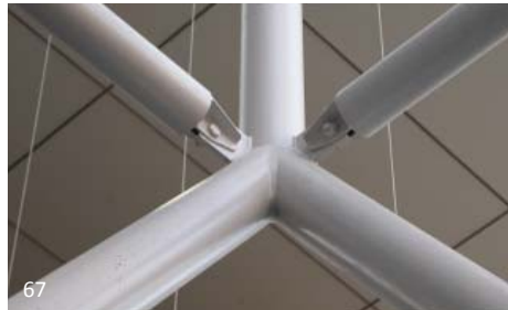
Fig. 4.1. This project uses mechanical pipe instead of HSS as the three dimensional nature of the structure made positioning seams out of view difficult and a seamless appearance was important. Grinding of the seams would have been prohibitively expensive as well as time consuming.
