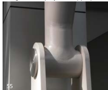
55 Fig. 2.4A The grinding of these welds incurs a cost premium but is necessary for the seamless look of the connection. This is not universally necessary, especially considering the viewing distance of AESS 2 elements. This treatment should be saved for AESS 4 Characteristic 4.3 Surfaces filled and sanded, where the elements are in close viewing range and sometimes able to be touched.
