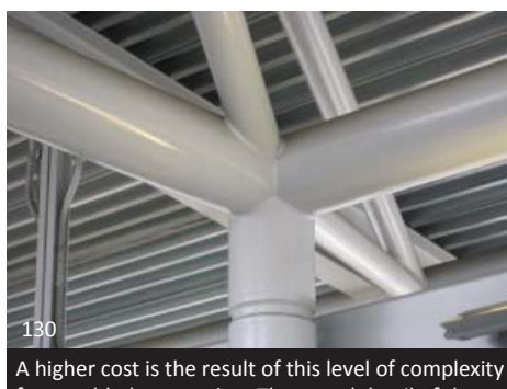
130 A higher cost is the result of this level of complexity for a welded connection. The reveal detail of the connection of the upper structure to the column makes the connection simpler to erect.
