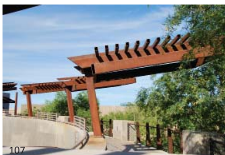
107 Care must be taken in detailing weathering steel to avoid having the natural oxidizing process create stains on the surfaces below the material.
