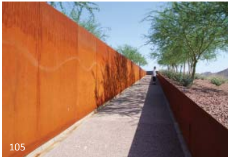
105 This garden wall is made from weathering steel. Although durable in appearance, you can see the destructive markings on the surface made by users of the space. It is essential to detail these types of installations so that the run-off water does not stain surfaces below the wall.
