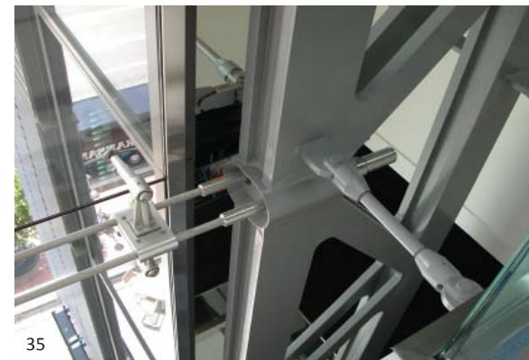
35 The Newseum in Washington, D.C. by Polshek Partnership uses a combination of AESS 4 quality steel with some custom specialty elements in this inventive support system that forms the support and wind bracing for a large mullionless glazed wall at the front of the building. Stainless steel brackets hook on to parallel tension supports that are braced on either side of the façade by these vertical trusses that are fabricated from parallel sections of plate steel.
