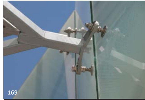
169 Alignment issues between the glass and steel support frame are taken care of by levelling mechanisms that are part of the glass connection system. These are located on the rear of the canopy so not visible from the front, allowing for clean lines and uniformity on the public side of the system.
