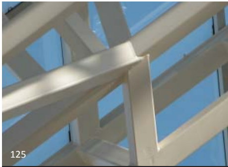
125 Complex connections using square HSS members are very difficult when it comes to alignment. Circular members are more forgiving. This connection is located on a high level skylight, so the alignment issue is not really visible.
