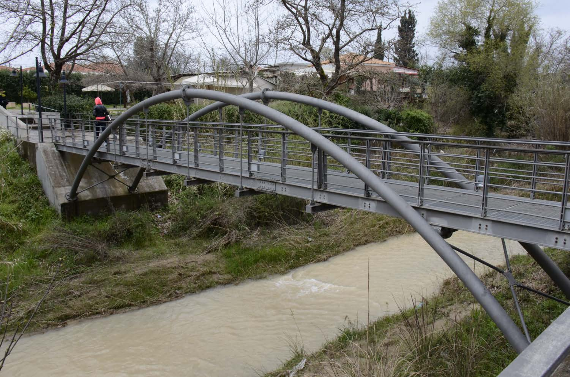
Bridge coated with a zinc rich paint which is holding up well but the bolts are inferior and are rusting.
