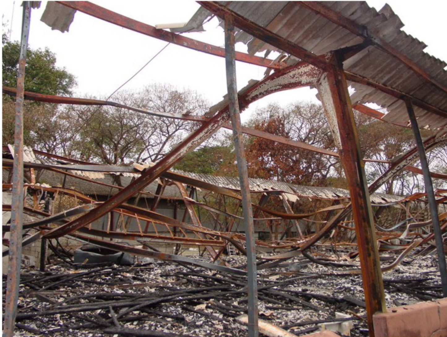
Galpão USP - 2002 - São Paulo - steel beams have melted
