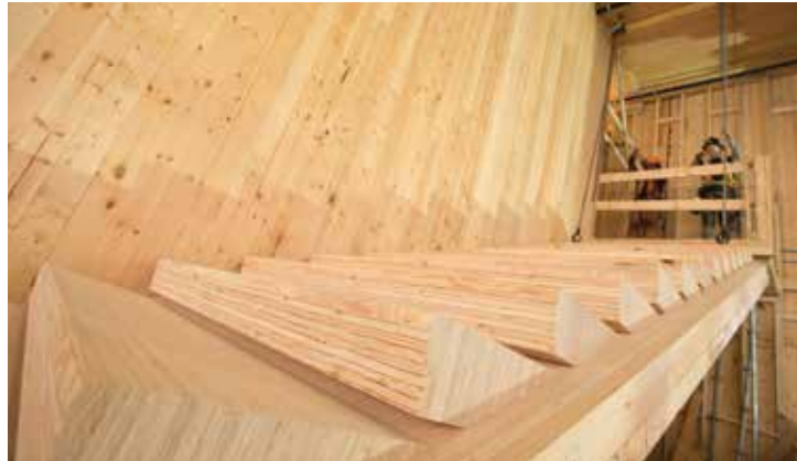
Building the feature stair: installation of LVL risers on the inclined LVL stringer panel
