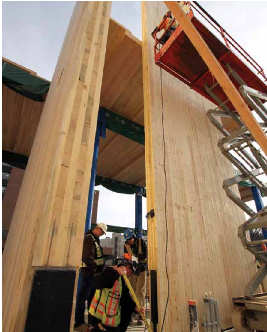
CLT core panel showing a tie-down connector
