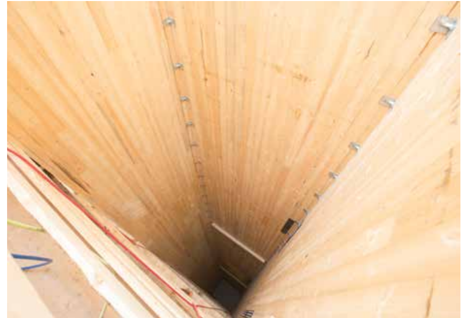
The CLT elevator shaft did not require any special acoustic treatment as it is not adjacent to noise sensitive areas
