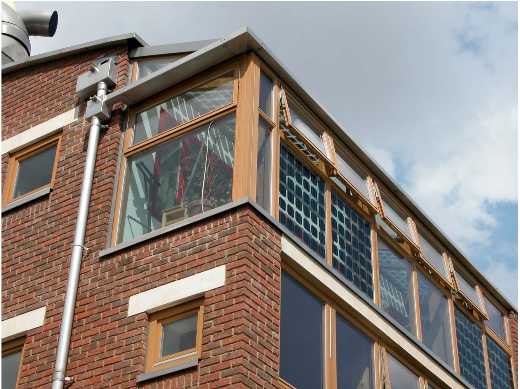
Thin PV integrated into the glazing at BedZED
