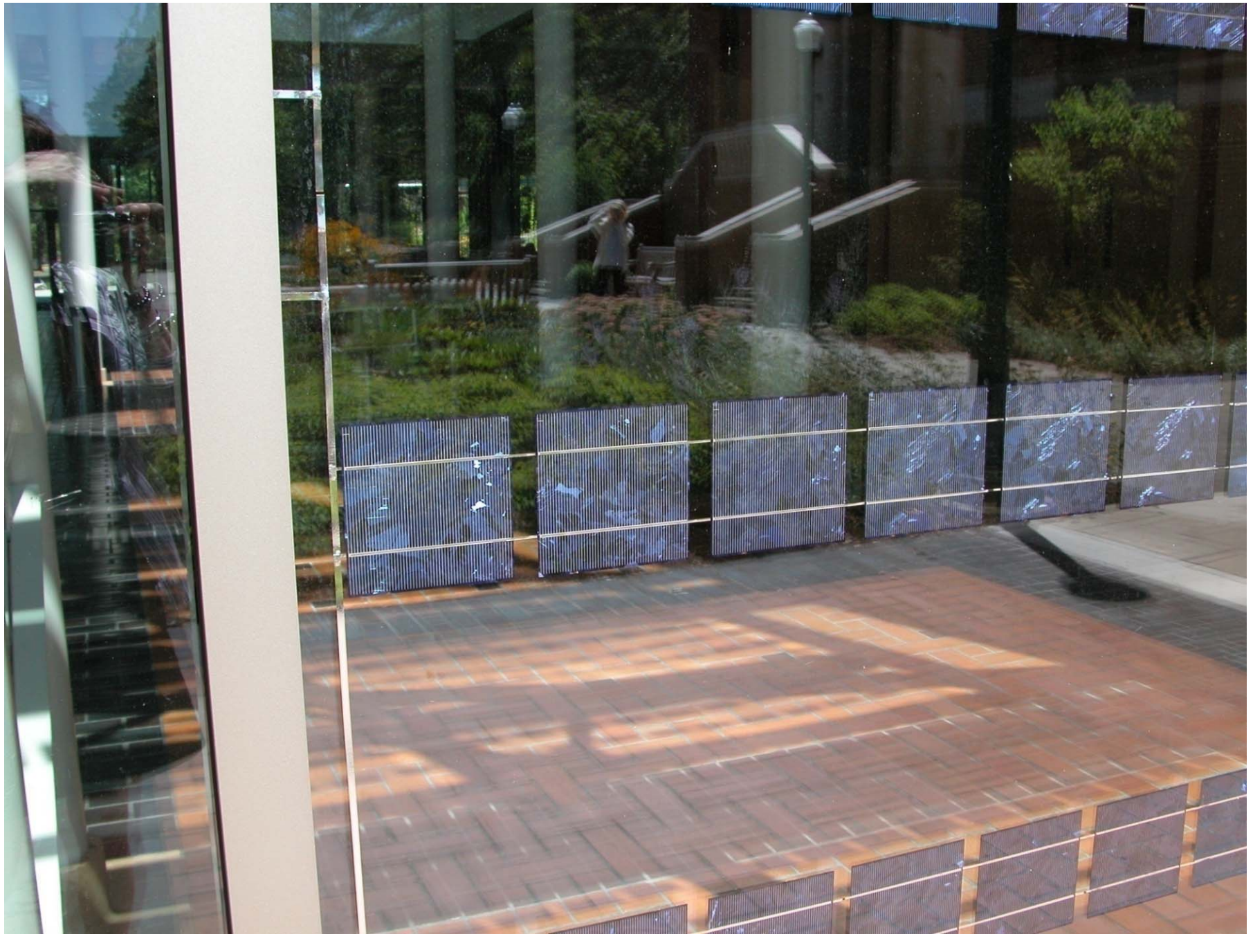
Thin PV integrated into the glazing at Lillis School of Business, U of Oregon
